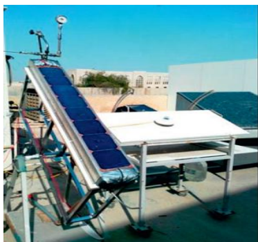
Fig. 2- Converging channel cooling for solar PV at site [4]
