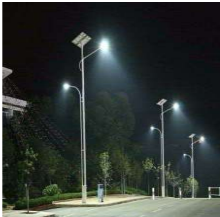
Fig. 1. Smart Street Light System
