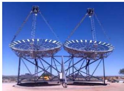
Fig 3 -Grid Solar Plant System
