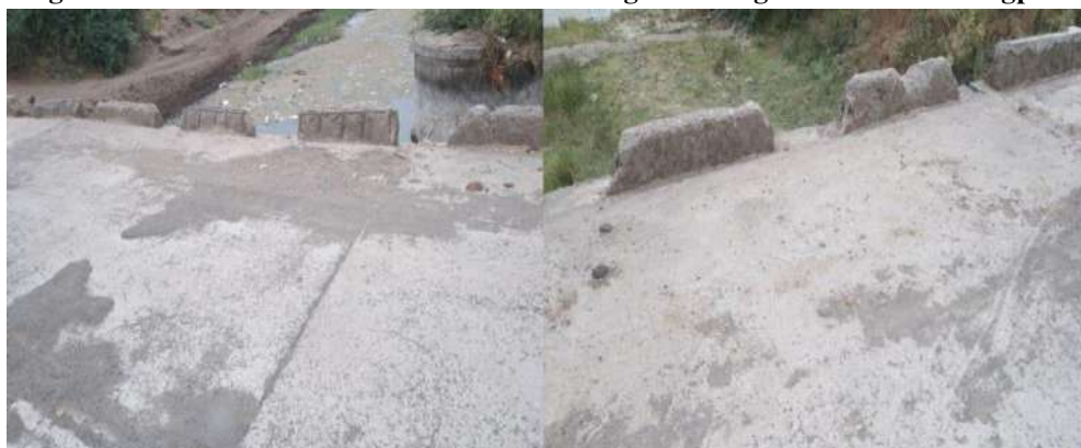
Figure 6: Damage Wheel Guard and Reflectors
