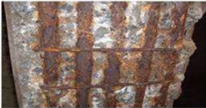
Fig.2 Corrosion in RC structure
