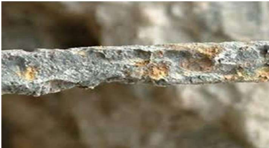
Fig.1: Corrosion in reinforcement
