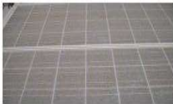
Fig. 3: Solar module covered by heavy layer of dust accumulated before cleaning
