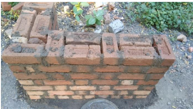
Fig. 5- Improper filling of mortar
