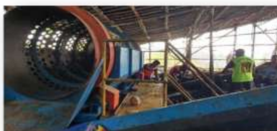
Figure 2.2: Unusable Machine at Malad Plant
